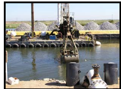
CCWD and Town of Discovery Bay Twin Outfall Construction in Old River
