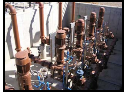
Town of Discovery Bay RAS/WAS Pump Station
