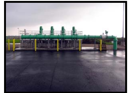
Town of Discovery Bay 4.2 MGD Export Pump Station
