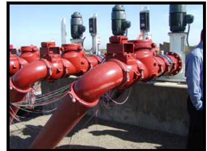
Town of Discovery Bay 6 mgd Effluent Lift Station
