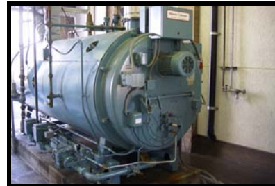
City of NAPA 3 Million BTUH Boiler
