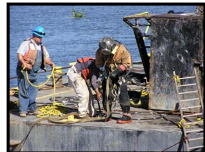
CCWD and Town of Discovery Bay Twin Outfall Construction in Old River
