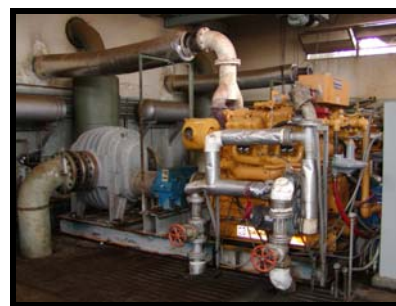
City of West Sacramento Digester Gas Cogeneration Emissions Control Project
