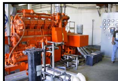
City of NAPA 600 kW Digester Gas Cogeneration System
